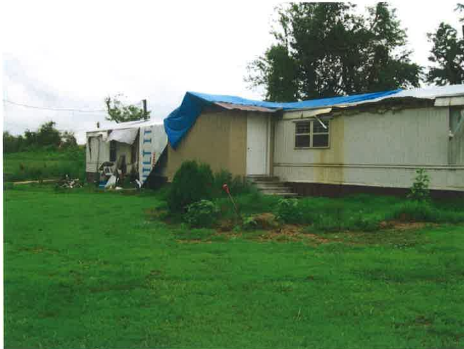
Trailer demolished in Lincoln County tornado
